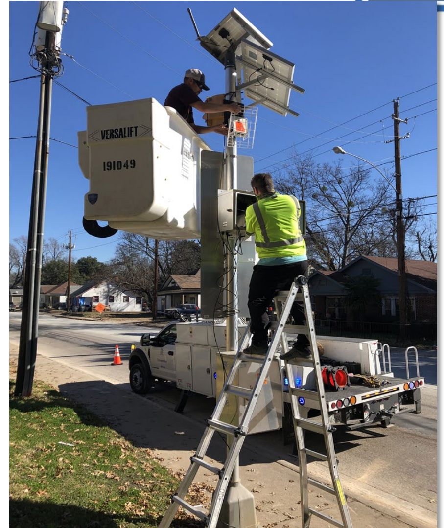
Air Quality monitor installation at Exline Recreation Center
