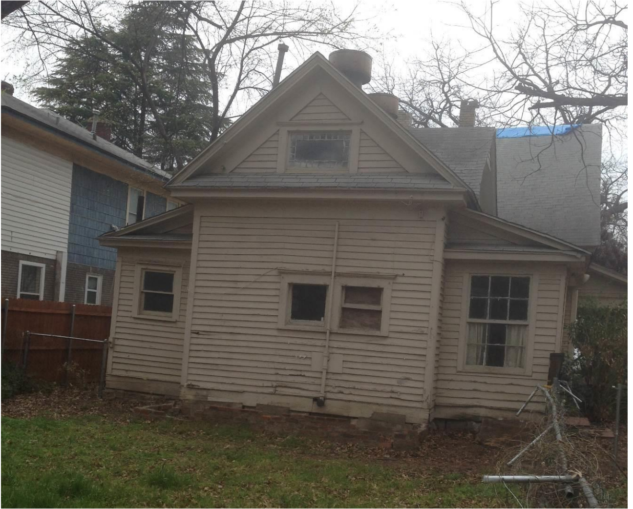
Rear of the main structure in April 2014 showing the wood skirting and siding intact. Photo submitted by applicant at time of Routine Maintenance request to replace no more than 10% of the wood siding with wood siding.
