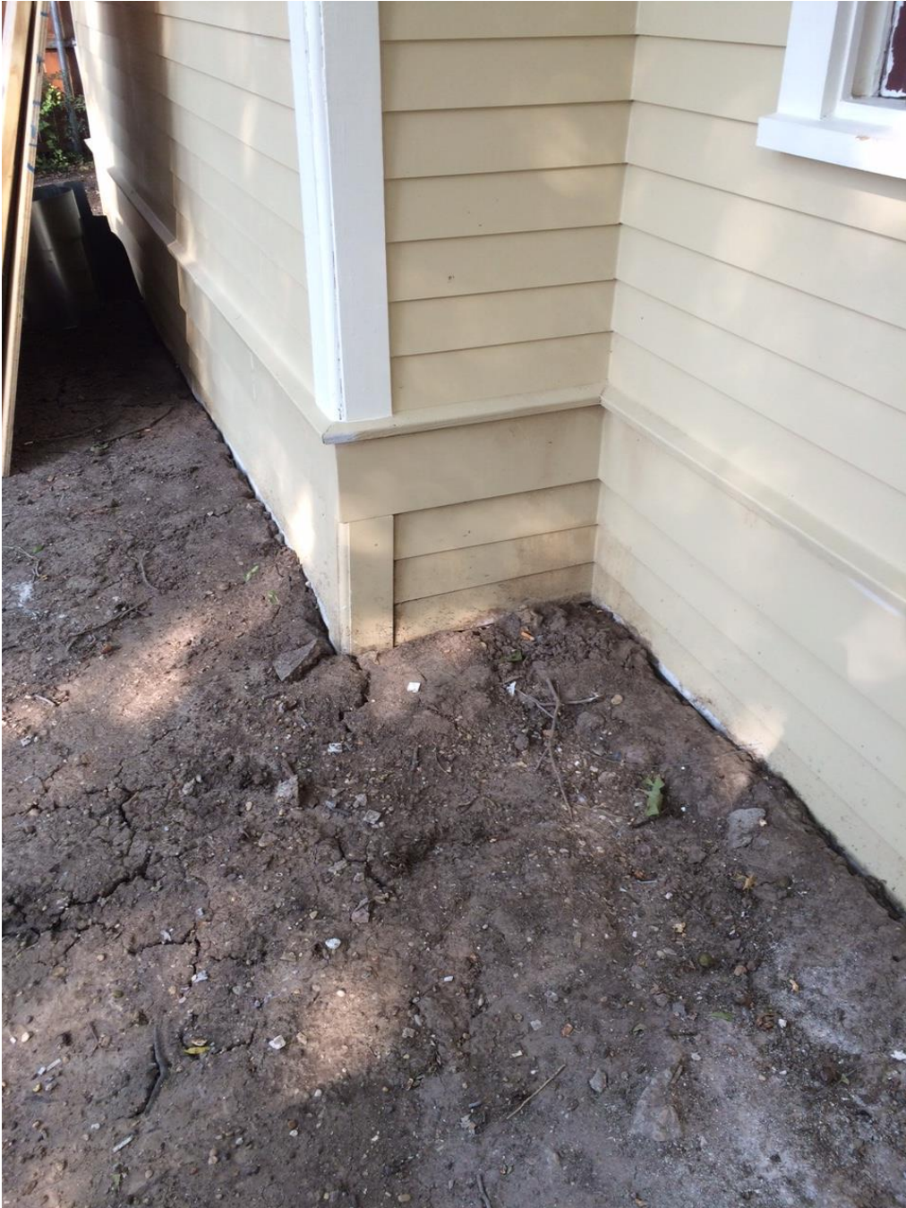
July 2015 - Hardiboard skirting and siding installed without a Certificate of Appropriateness. Photo by Code Enforcement at time of Stop Work Order.
