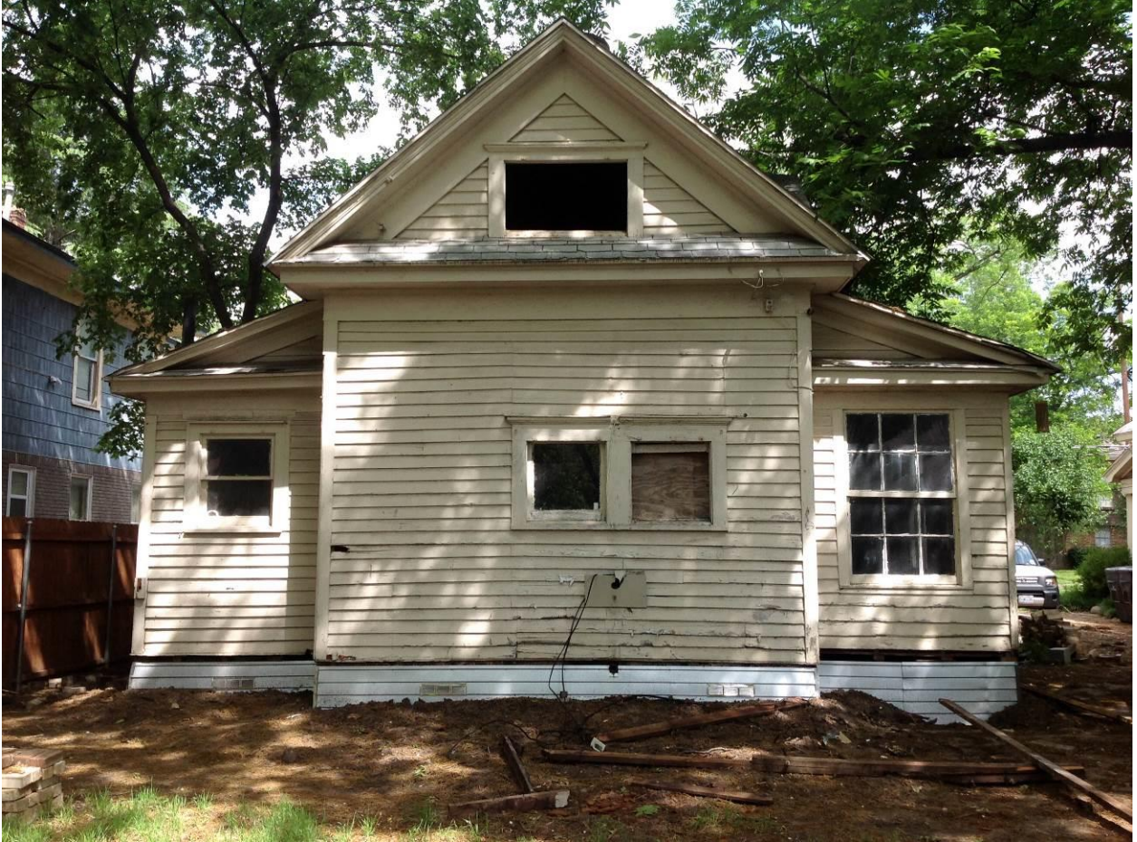
Rear of the main structure in August 2014 showing the wood skirting replacement with metal skirting and wood siding intact. The metal skirting was installed without a CA and Denied without Prejudice by the Landmark Commission .Photo by Code Enforcement at time of Stop Work Order.
