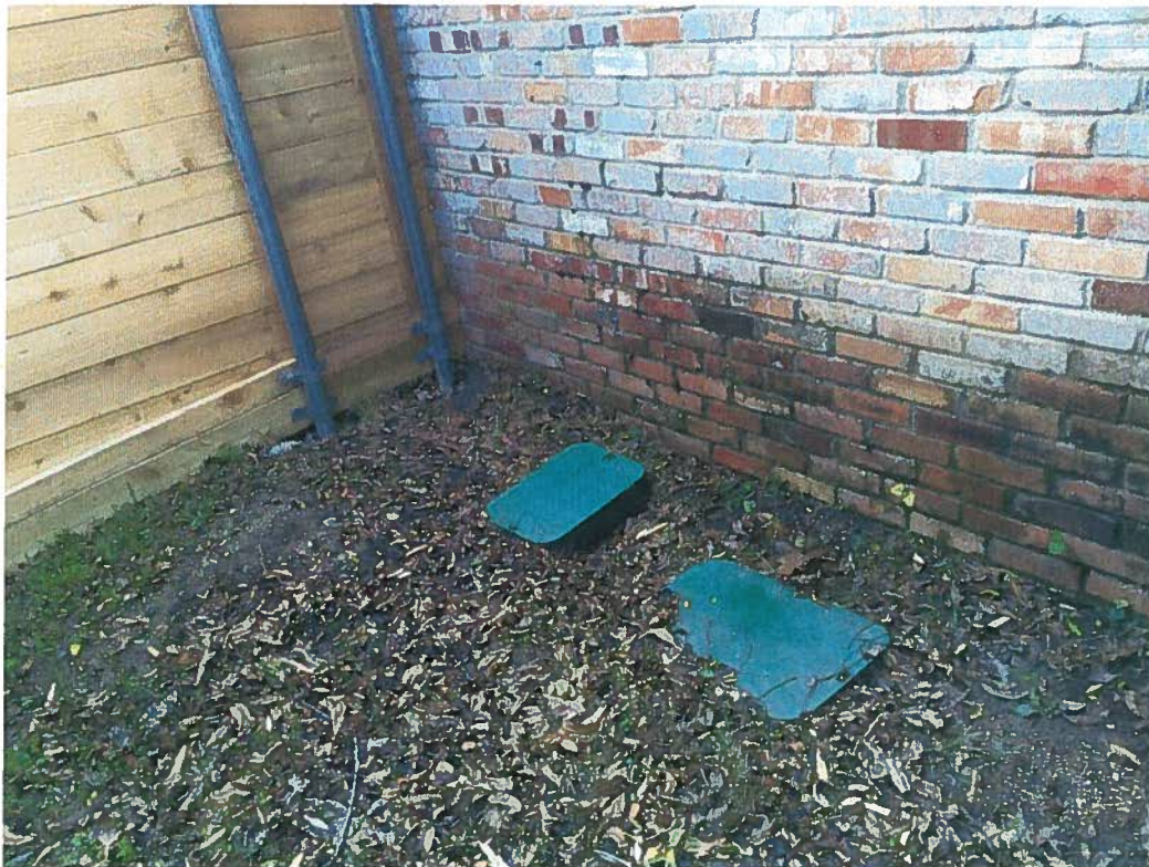
Water & sprinkler control boxes located on side near front of house.
