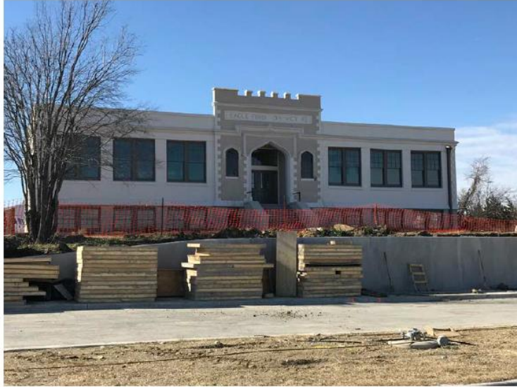
East façade at Chalk Hill Road, looking west. This shows the new concrete retaining wall at cut into the site in conjunction with construction at Chalk Hill Road. January 28, 2019.
