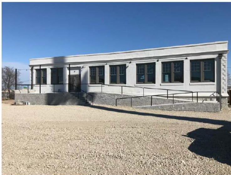
West (rear) façade, with new stairs, accessible ramp and porch at new rear door. January 22, 2018.
