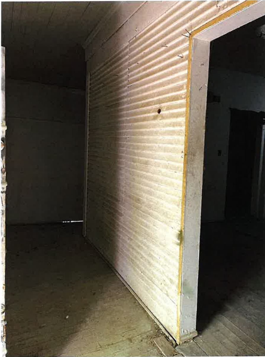
Figure 19 - Detail view revealing an understanding of fenestration that is evident within the space occupied by the wrap-around porch (photograph taken July 25, 2022)
