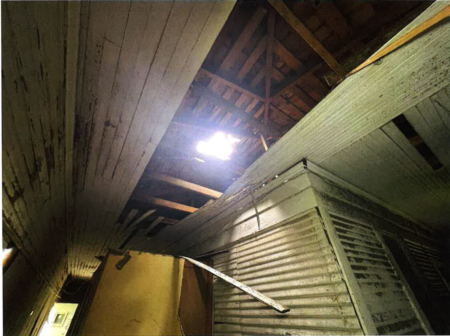
Interior View Porch ceiling damage SE corner looking west
