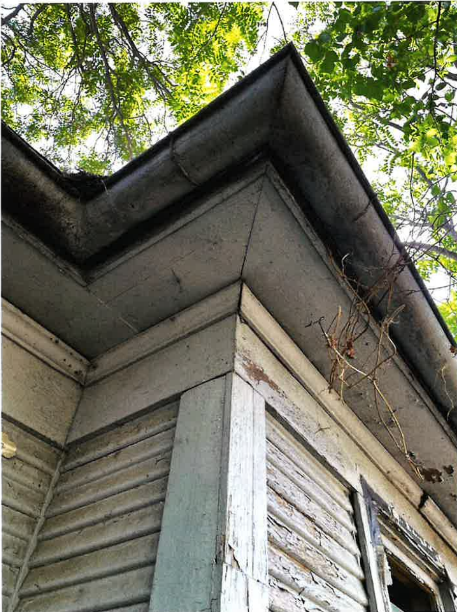
Figure 8 – Detail view showing the character of workmanship that is evident (photograph taken July 25, 2022)
