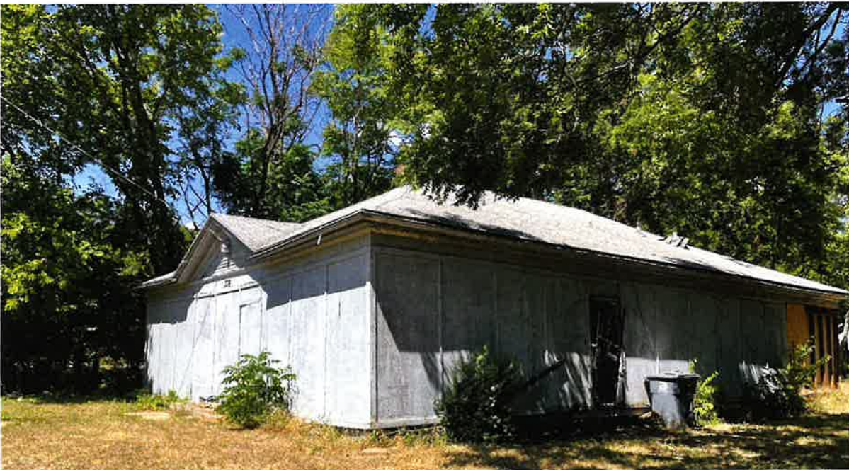
Figure 15 - View of the subject property as seen from the southwest corner (photograph taken July 25, 2022)
