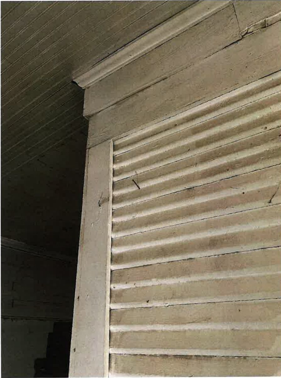
Figure 18 - Detail view showing the character of workmanship that is evident within the space occupied by the wrap-around porch (photograph taken July 25, 2022)
