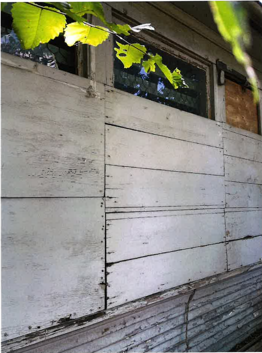
Figure 22 - Partial view of the north side projecting bay showing evidence of fenestration patterns and character (photograph taken July 25, 2022)
