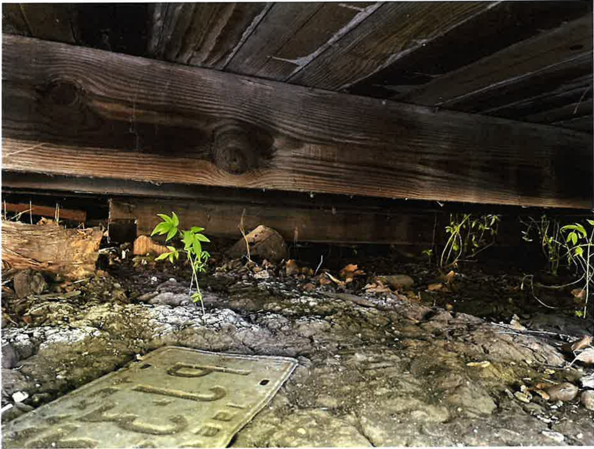
Figure 23 - View gained from one of several areas showing the underside of the structure (photograph taken July 25, 2022)
