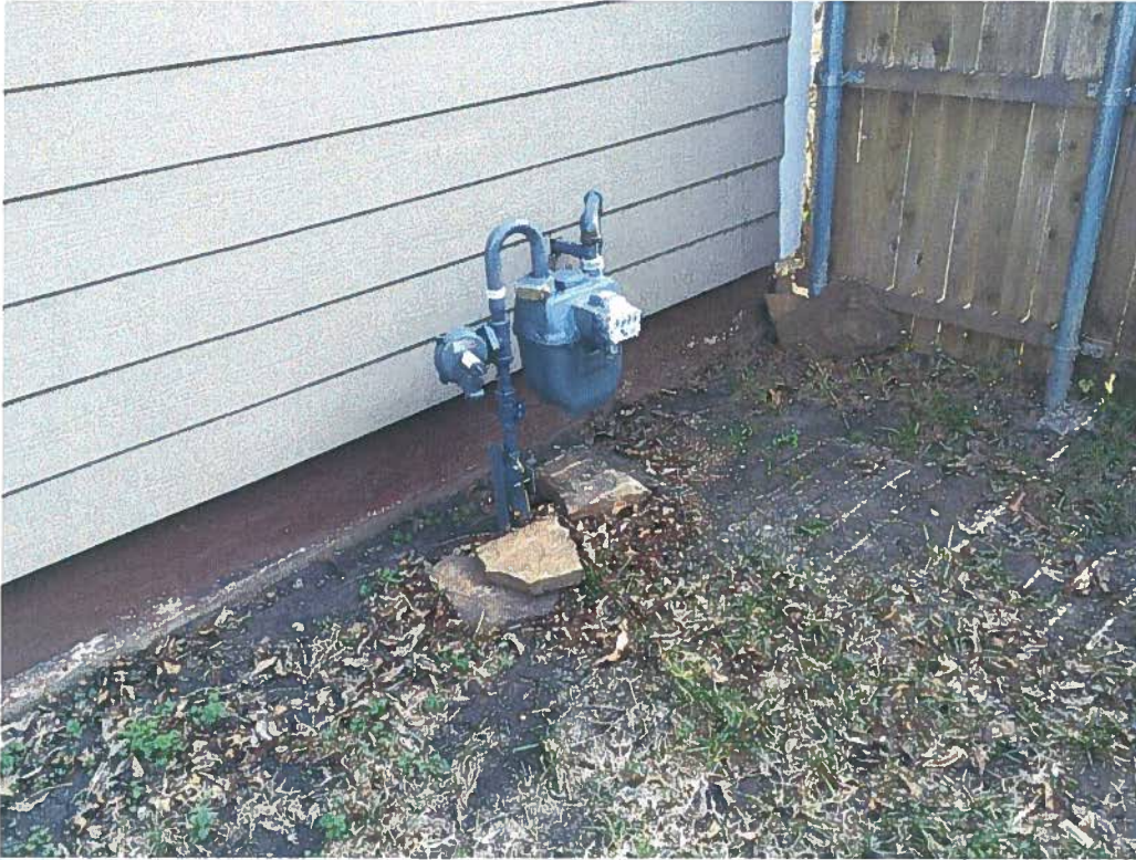
Gas meter located on side near front of house.
