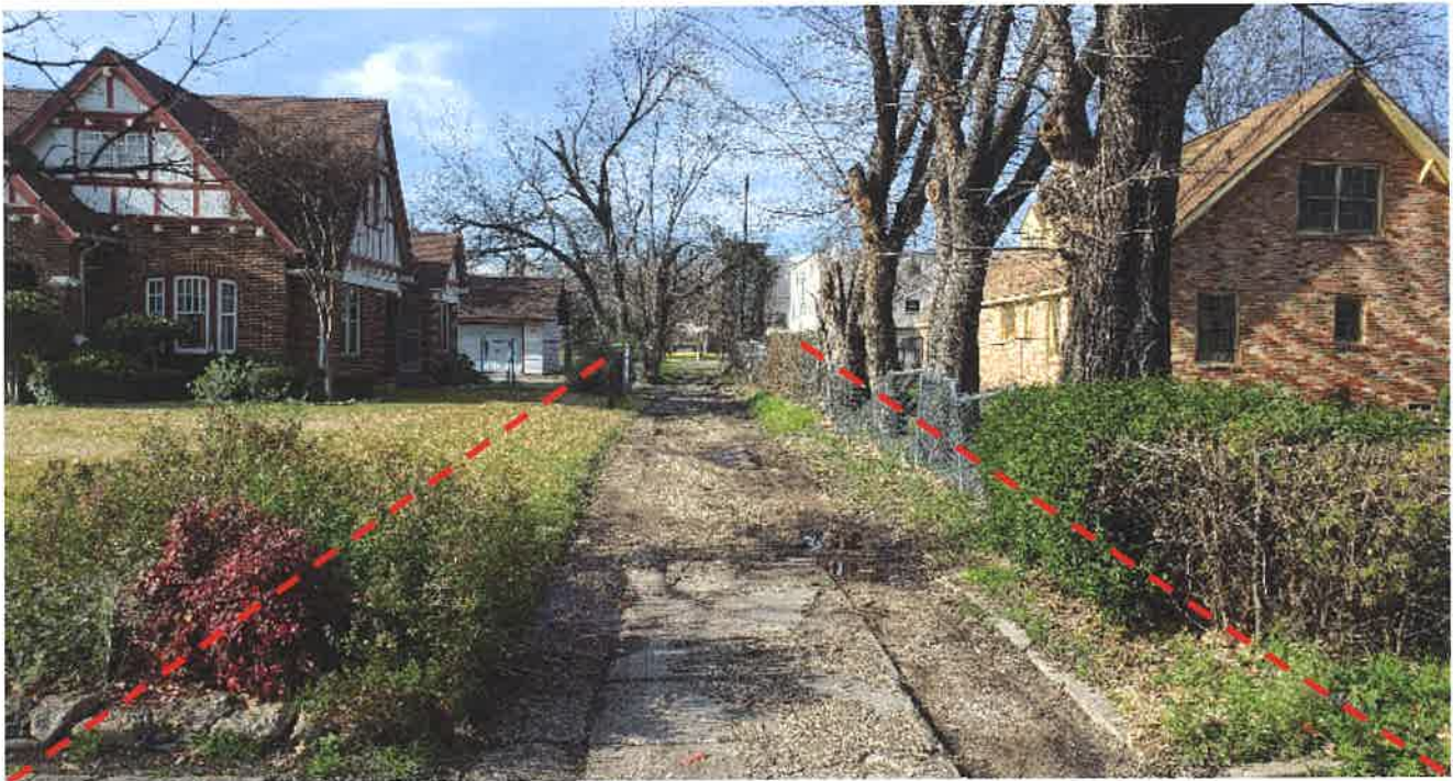
A4: Pictured: North facing view of Myrtle Walkway easement (sidewalk) at Park Row Ave (approx. 55 yards south of 2634 Al Lipscomb Way ).
