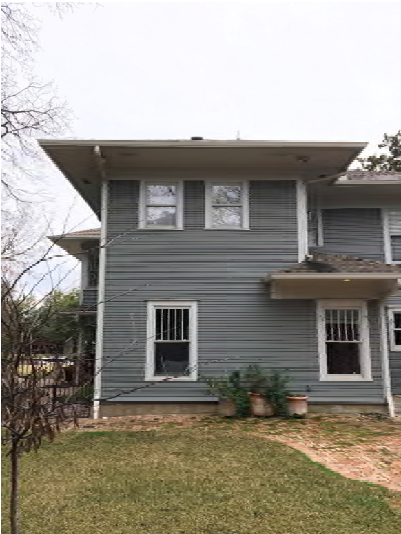
View of existing rear façade modified during previous remodel by different owner.
