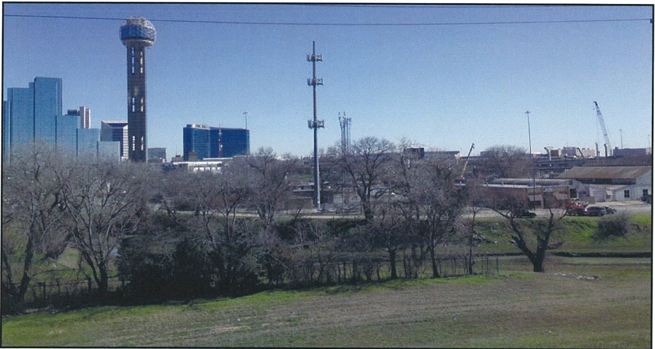
Extended 150' Monopole Tower
