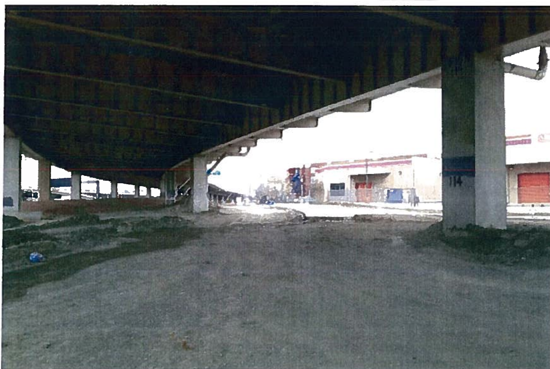
View north along new Cesar Chavez alignment (under construction); existing Public Storage facility on right, request site just beyond, then Live Oak Lofts in background.
