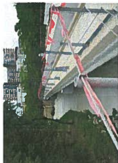
D Turtle Creek Bridge View of Turtle Creek Bridge showing construction progress.
